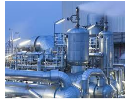
Steam Methane Reforming - Hydrogen Production (Air Liquide, 2022)
