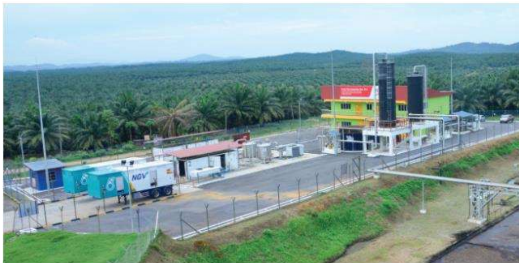
Figure 24. Bio-CNG plant at Sg Tenggi Palm Oil Mill in Malaysia
