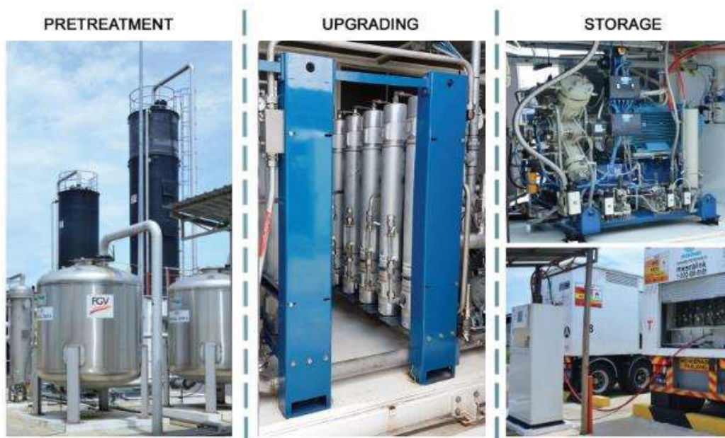
Figure 25. Main operation unit of Sg Tenggi Bio CNG plant
