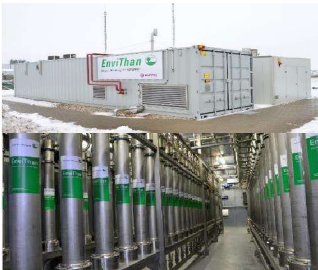
Figure 23. Sachsendorf biogas upgrading plant using membrane system
