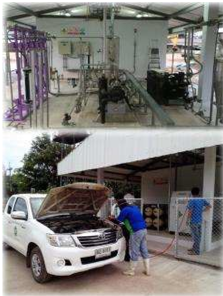
Figure 26. Bio-CNG plant in Khon Kaen University, Thailand
