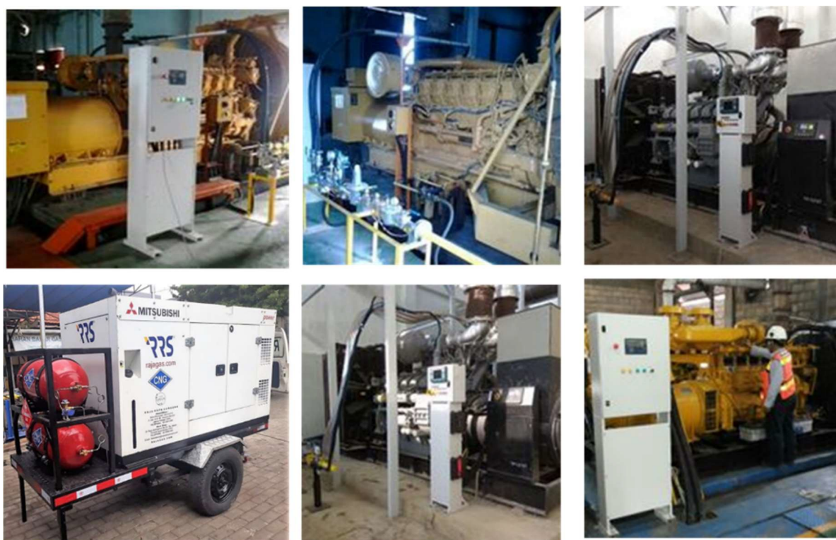
Figure 20. Dual fuel or dedicated system for generator
